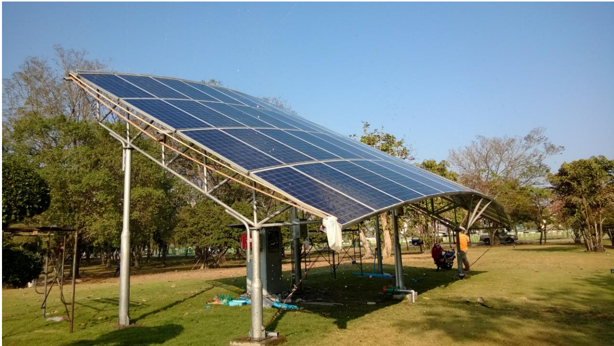
Figure 7: Other side of 10kWp photovoltaic system.
