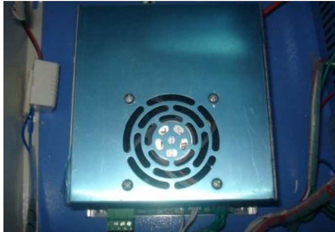
Figure 3.3 The power supply
